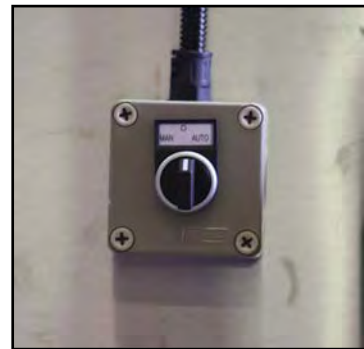
Manual Off/Auto switch install on ITS
